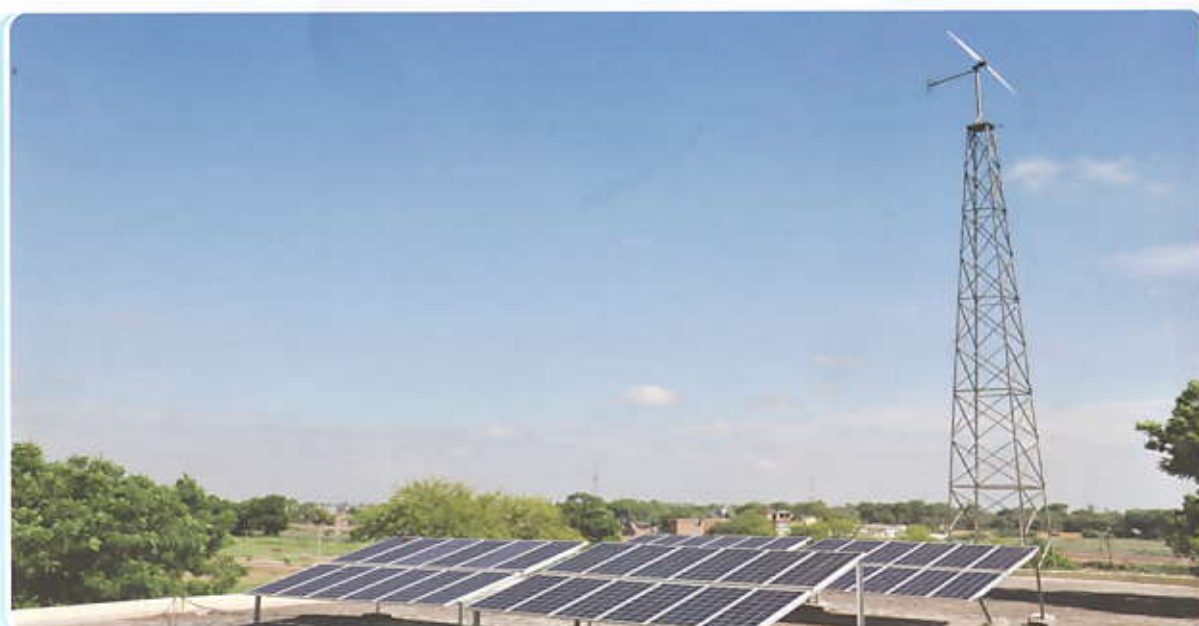
Solar Photovoltaic Panels and a Wind Mill
